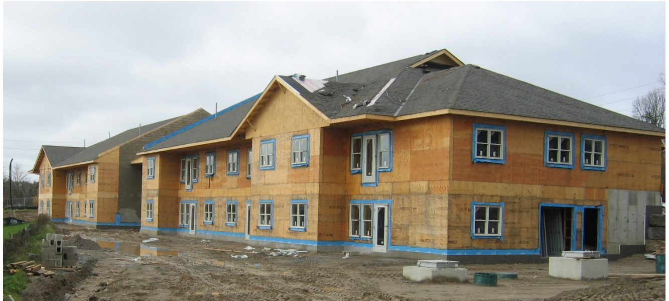
PHOTO TAKEN OF THE TWO STOREY REAR BUILDING ELEVATION AT FINAL STRUCTURAL FRAMING INSPECTION.
